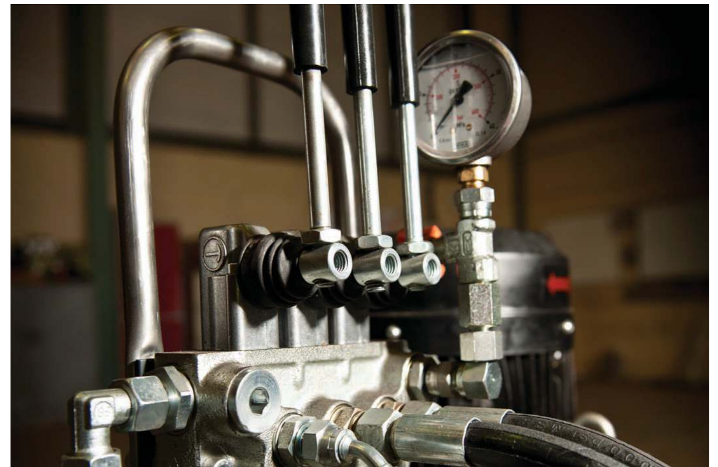
Hydraulic Curtain Adjustment and Frame Opening
