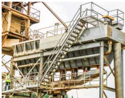
CLASSIFYING TANK WITH STAIRWAY
